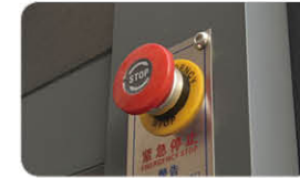
紧急停止开关 Emergency stop switch
